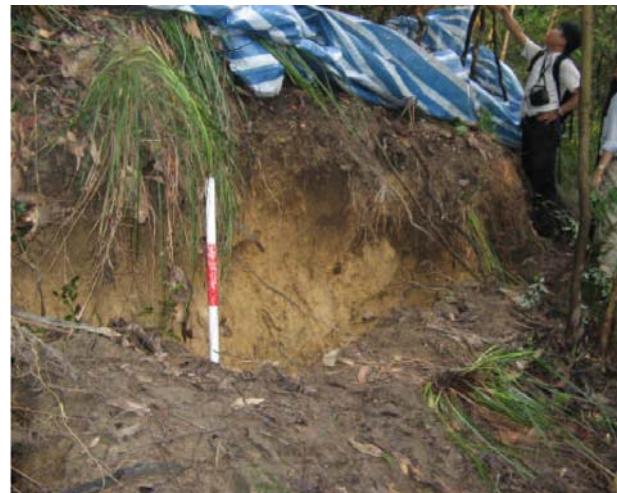
Figure 15 – Displaced landmass revealed in site inspection
